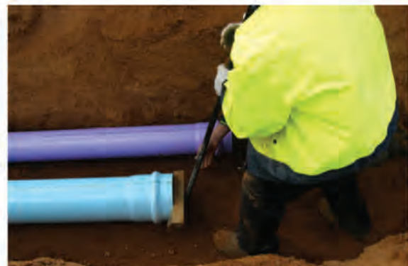
Figure 7.8: A DN150 ApolloBLUE™ pipe is being joined by pushing with a crow bar. Note: the pipe socket is protected from possible damage with a block of timber.
