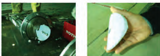
Figure 7.16: Use of a hole-saw cutter in the tapping machine results in a cleanly cut coupon
