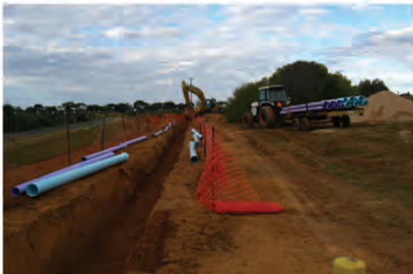
Figure 3.1: A combined trench installation using blue DN100 and purple DN150 ApolloBLUE™ for a dual water supply at Bamera, South Australia
