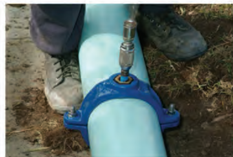
Figure 7.11: Taptite polymeric coated DI tapping band installed on an ApolloBLUE™ water main. Shown here is a brace and bit fitted with a hole saw being used for a “dry” tapping.
