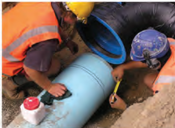
Figure 7.9: A new witness mark is being stencilled to take into account the ductile iron fitting socket depth.
