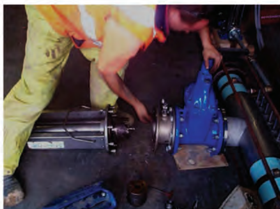
Figure 7.15: Live tapping of a DN150 ApolloBLUE™ pipe with a DN150 branch connection using a Crevet stainless steel flanged branch and flanged AVK gate valve.
