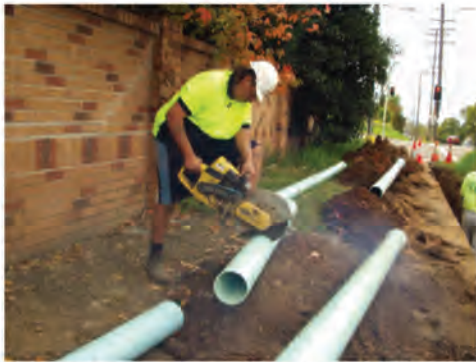
Figure 7.6: Powered disc cutter is being used to cut ApolloBLUE™ to length on site
