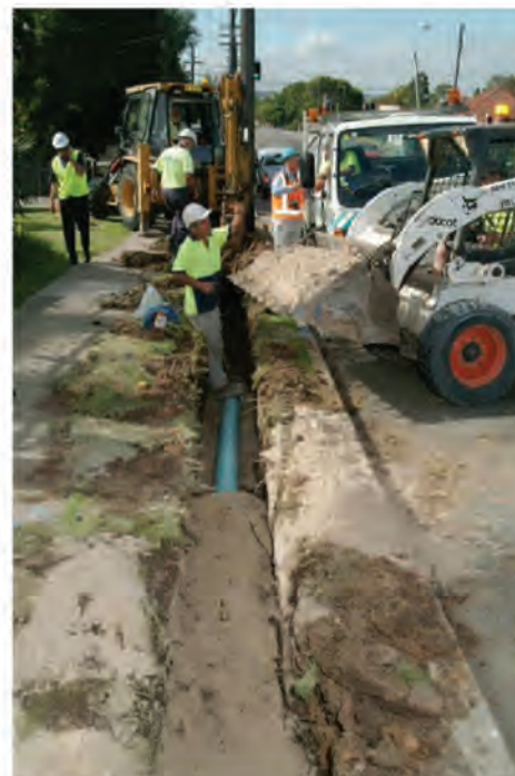
Figure 7.5: A granular embedment material should surround pipes and be adequately compacted in the side support zone before excavated material is placed into the trench.
