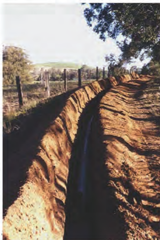
Figure 7.8 - DN 150 PN 6 S1 RHINO™ pipeline laid on a curved alignment near Broke, NSW
