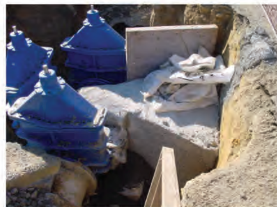
Figure 6.2 - Concrete thrust block, correctly oriented to transfer the hydraulic thrust to the specially trimmed undisturbed soil of the vertical
