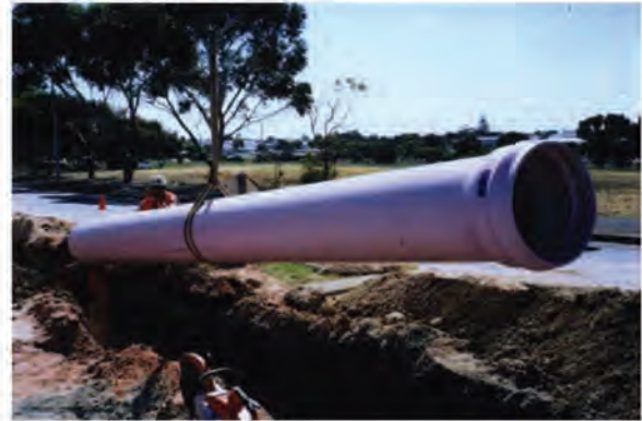
Figure 3.1 - Iplex DN450 PN12 Series 2 PVC-M purple pipes for recycled water at Willunga, South Australia.
