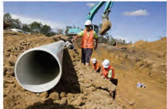
Figure 1.1 - WHITE RHINO™ PVC-M Pipes being installed at the Wimmera Mallee Pipeline Project, Victoria.
