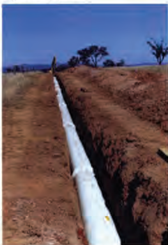
Figure 7.3 - DN450 PN 9 WHITE RHINO™ pressure pipe for irrigation supply in Hunter Valley, NSW
