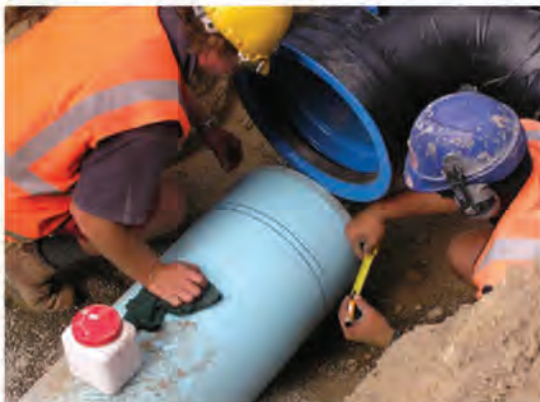
Figure 7.6 – New witness mark is being stencilled to cater for the ductile iron socket being used.
